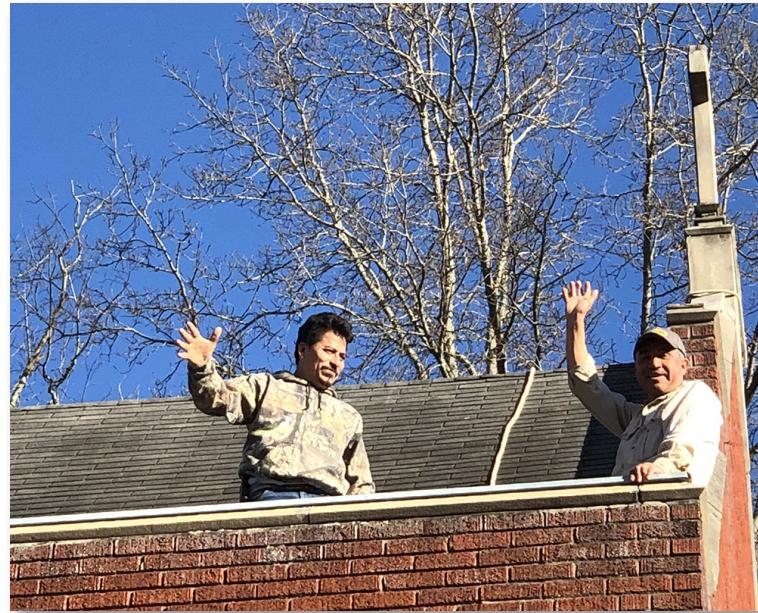
Roof repair and renovation work on the historic St. John the Evangelist Church in Waynesville is set to begin April 22 and, weather permitting, will be completed by Aug. 7.
